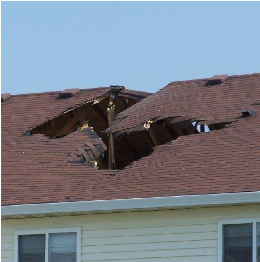
Close-up of gaping hole from helicopter crash directly into the home
